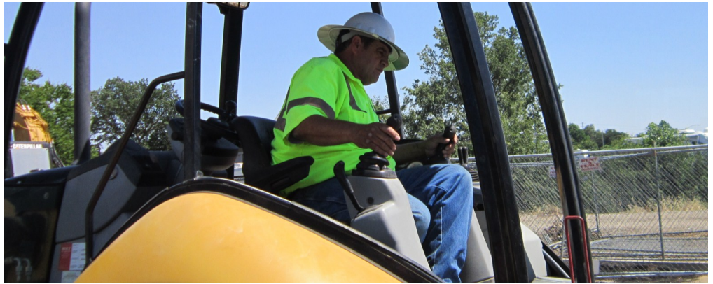
Richard Salas oversees the moving of water lines to make way for the new Elk Grove pedestrian overpass.
